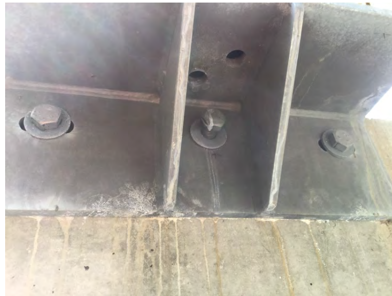
Loose riser bolts
